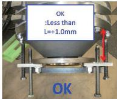
Figure11 OK Circlip not missing
